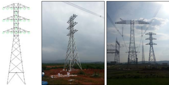
Fig. 1. Shielding wire support tower
